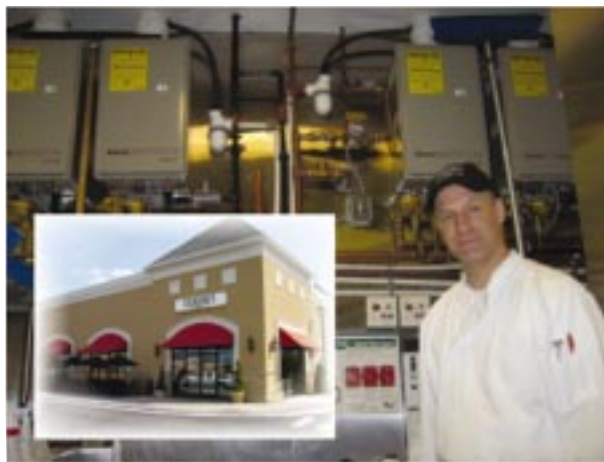
Chef/Owner Bill Nixon shows off his space saving gas tankless water heating system.
